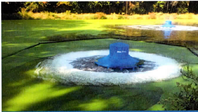
City of Cushing, Blue Frog Aeration System
