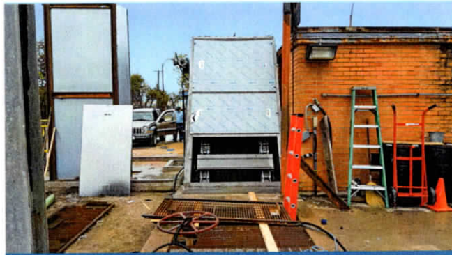
City of Ennis, Mechanical Bar Screen
