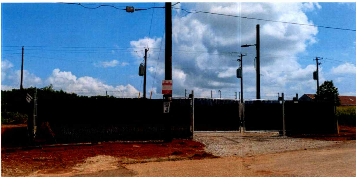
Sunnydale Lift Station – Exterior View
